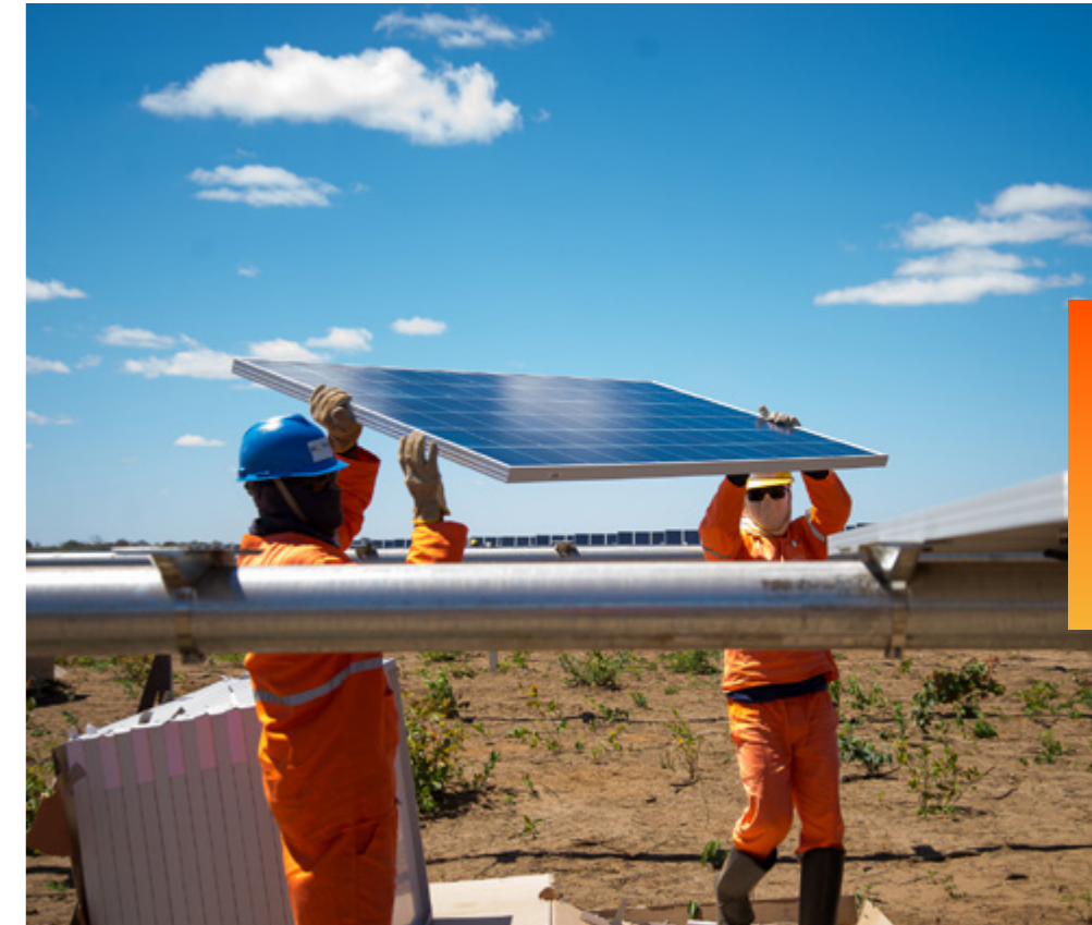
Atlas Renewable Energy collaborators mounting solar panels in our Juazeiro Solar Plant in Brazil
