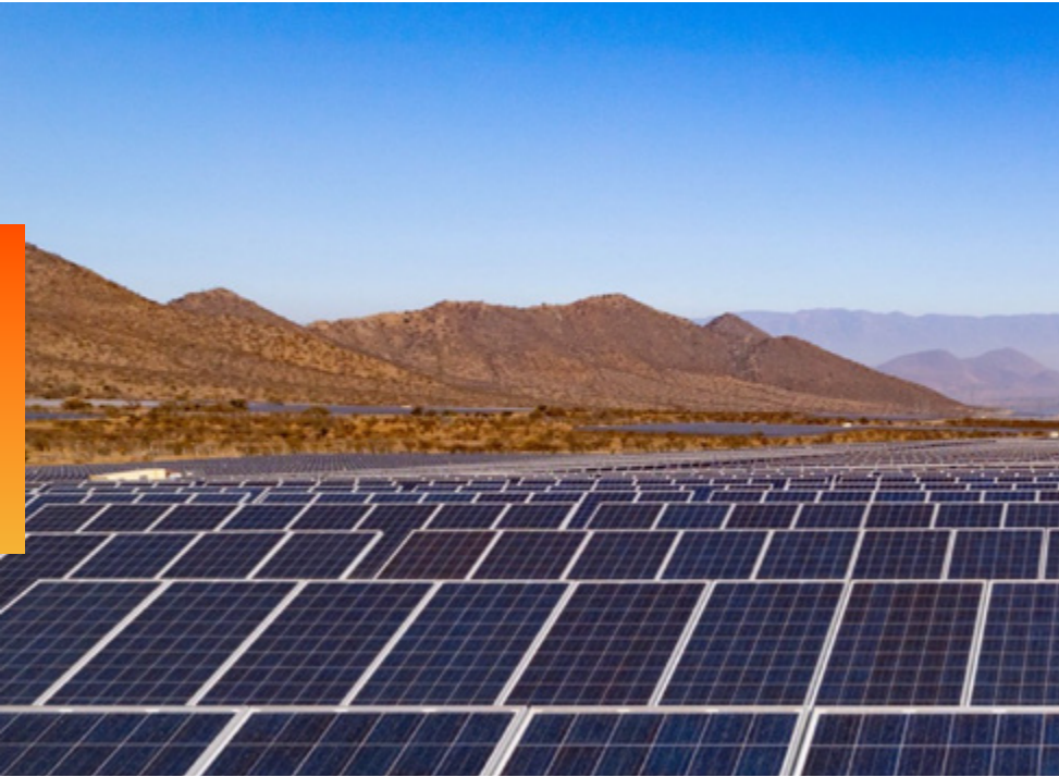
Quilapilun Solar Plant in Chile's Antofagasta Region
